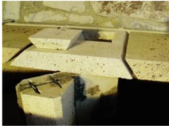
FIGURE 8.49. The inner life is capped with 11.4-inch refractory slabs. The middle slab is fully supported from below, but the others are not. The skew cuts will provide structural support as needed. At top is a cleanout access. Again, skew cuts will guarantee that the cleanout “door” can never fall into the heater. Gravity and clay mortar will guarantee, as well, a gas-tight seal.
