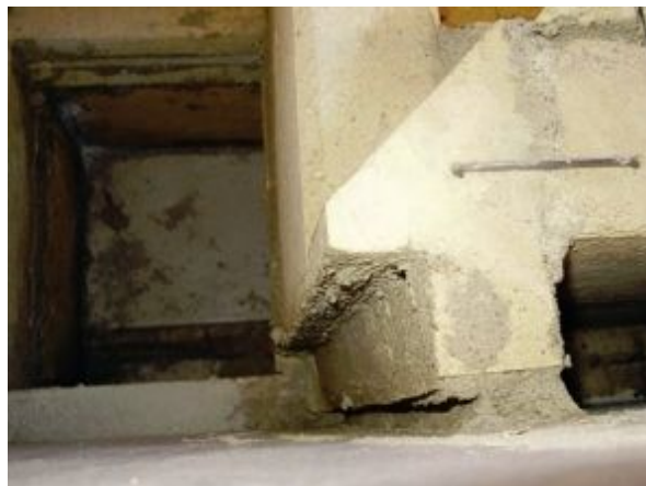
FIGURE 8.31. A notch at the corner of the outburn will accept the lining of the first flue, yet to be placed. The notch guarantees that the refractory lining can never fall out of place.
