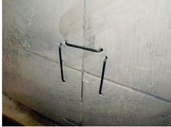
FIGURE 8.28. The backside (inner-life side) of the soapstone, showing metal clips binding the stone together both horizontally and vertically.
