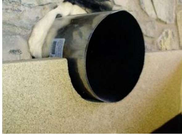
FIGURE 8.30. The insulation board is cut around the stainless-steel flue. In this project, an uninsulated metal 8-inch flue was relined with an insulated 6-inch flue.
