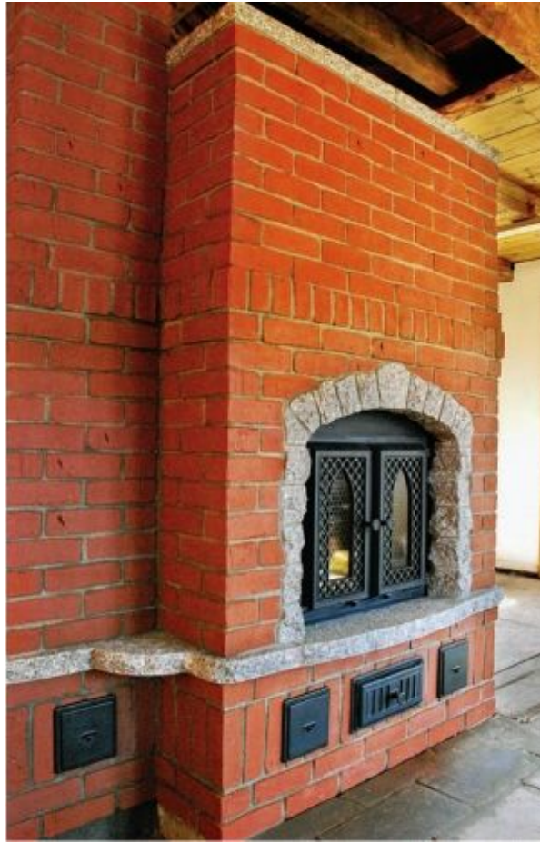
FIGURE 9.19. Three cleanouts are visible on the lower part of this beautiful brick heater; one is on either side of the ash box door, and one is at the base of the chimney on the left. Photo courtesy of Maine Wood Heat Company.
