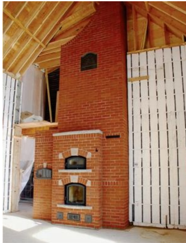
FIGURE 4.17. This massive red-brick masonry heater has granite accents. The room is yet to be finished, but the towering chimney will be entirely visible when the cathedral ceiling is done. Notice that this heater has two bakeovens, one above the main firebox and one to the left. Photo courtesy of Maine Wood Heat Company.
