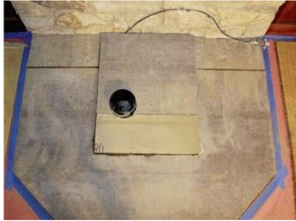
FIGURE 8.12. The project under way. Visible is a 6-inch-diameter air-supply duct at left middle. The cable attached to the stone wall is the control to open and close the gasketed air-intake damper. The working surface is cement board over Foamglas insulation to minimize heat transfer to the floor below.
