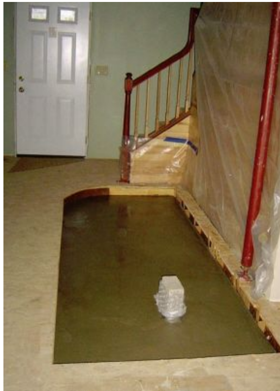
FIGURE 9.2 (left). Concrete is poured into the formed cavity for a foundation capping slab. Notice steel rebar tied together on 6-inch centers. The protruding insulation-wrapped wood in the foreground is to form a passageway through the poured slab for dumping ash into the foundation cavity below. | FIGURE 9.3 (right). The concrete pour is complete. Photos by Julie Cline.
