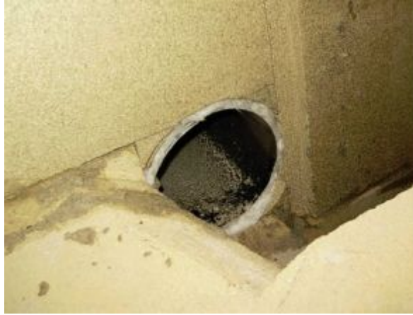
FIGURE 8.42. Another skew cut aids the final exhaust trip to the chimney connector. The chimney connector has been carefully insulated to seal tightly.
