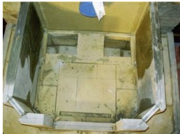
FIGURE 8.26. A view into the container. The cleaner plates forming a square in the middle are dry-set firebox floor elements. The floor will be two layers that are both set dry. These removable pieces allow access to clean the air-supply area that will, over the course of a year, accumulate some ash. The two rear flues are well defined here.
