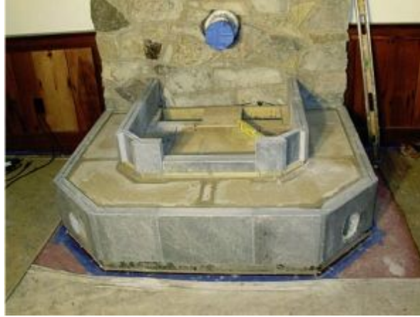
FIGURE 8.24. The entire set of bench flues is capped, and the first course of main-body soapstone is built. The shorter piece at front center is the base of the door opening. The soapstone overhangs the pieces on which it rests, forming a notch for inserting the granite, which was not yet available as this stage was reached.
