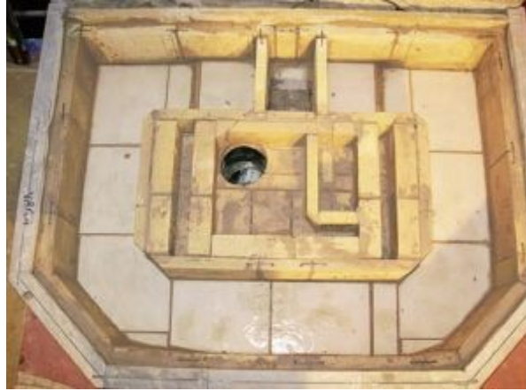
FIGURE 8.21. The support structure for the rest of the heater is built inside the container. The innermost rectangle roughly outlines the firebox floor to be built above it. The L-shaped pieces begin to outline the air-supply slot to the firebox. Notice that all plates lining the bench flues are “backed up” by additional bricks or plates. Inexpensive tile was used to line the floor of the flues. Everything was set in clay mortar and pinned together (though some pieces are not yet pinned in this and the following figure).
