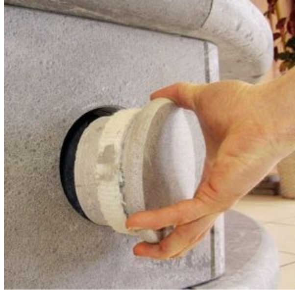
FIGURE 12.4. Soot plugs are removed annually to access the flues of the masonry heater. The access hole is usually large enough for a shop vacuum hose.
