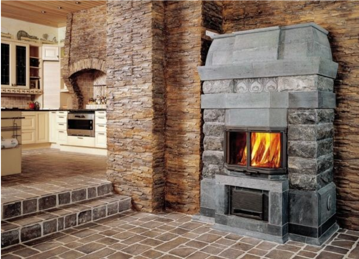
FIGURE 11.9. Tulikivi Corporation often suggests back-to-back firings in heaters like this. Notice how soapstone goes well with other stone and the tile floor. This heater features a panorama (multisided) door, large, rock-faced “bricks” that are carefully mitered at the corners, and sandblasted carvings in the stone centered above the firebox. Photo courtesy of Tulikivi Corporation.
