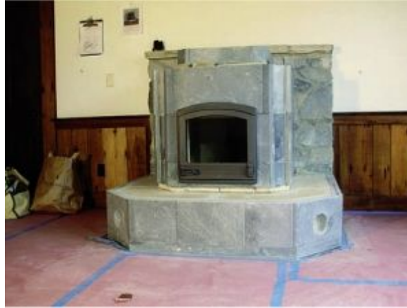
FIGURE 8.51. A door is installed, and the heater is ready for granite benches, trim, caps, accents, and final cleanup.
