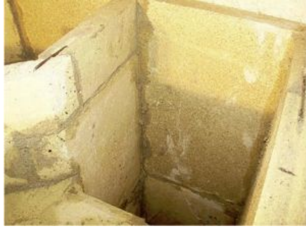
FIGURE 8.47. Another view of the updraft flue showing insulation board, half-lapped joint (lower left), and skew cut.
