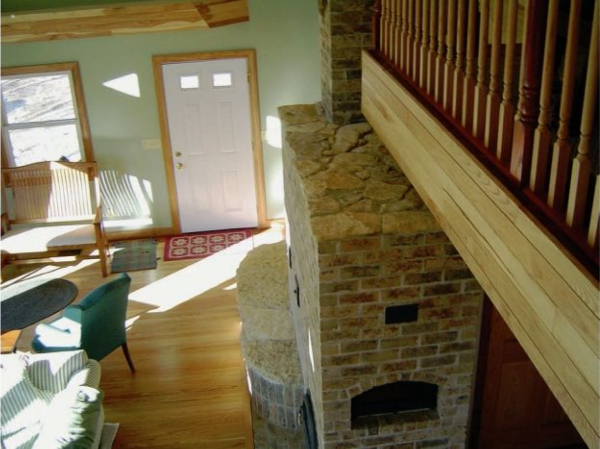
FIGURE 4.6. A view of a large masonry heater from a balcony. This heater is the sole heat source for a 2,500-square-foot home. The simple brick veneer is complemented by limestone—most of which was part of the paving outside various outbuildings on the property. Other views of this heater are in figures 3.5 and 5.1.
