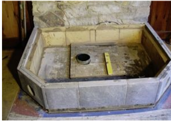
FIGURE 8.20. The base course of soapstone is in place, as is the first course of the inner flues. This first course outlines the heated bench and flues 3 through 9 of the heater—approximately 12 linear feet of flues. The exhaust will travel from the upper left of the picture counterclockwise to the upper right through this bench.
