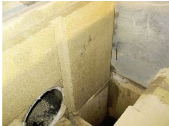
FIGURE 8.41. The right rear corner (vertical flue). More insulation board protects the stone-covered combustible wall behind. A sawn notch will capture another plate. Note also the skew cut on the lower right of the picture to aid the flow of exhaust into the upper flues.
