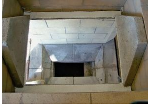
FIGURE 8.56. This view reveals the sloping firebox-floor pieces. In the foreground are two trapezoid-shaped elements of the Albie-Core that support the large, sloped dry-set throat pieces yet to come. Photo courtesy of Maine Wood Heat Company.
