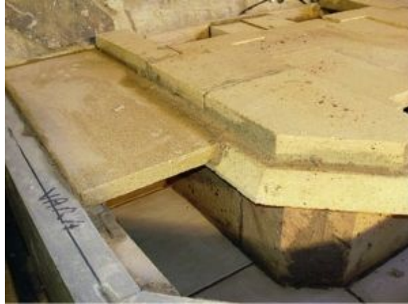
FIGURE 8.23. Two layers of plates over the base course further outline the inner life and form a structure on which to build the rest. The bench flues are being capped with Skamolex to reduce the temperature of the bench slabs. Note the skew cuts on the first layer of horizontal plates. The skew supports the Skamolex while providing a surface that is partially cantilevered over the bench flues to catch both the granite bench stones and the soapstone veneer of the rest of the heater.
