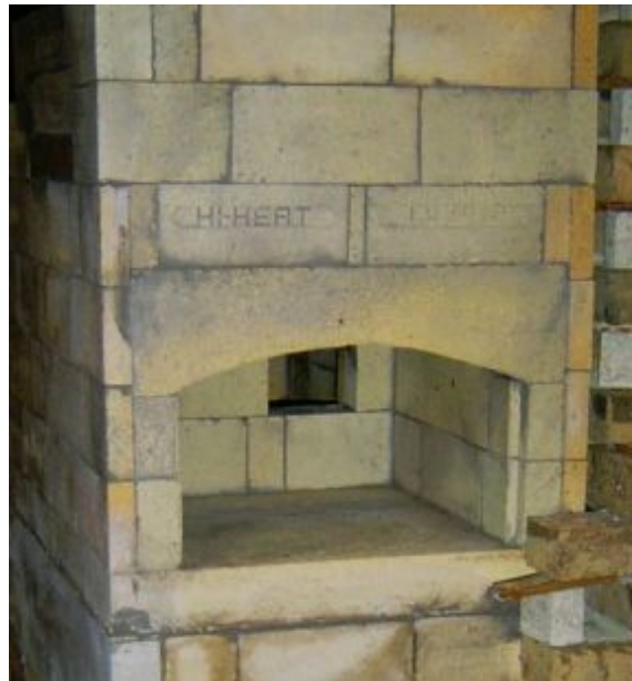
FIGURE 11.14. A white oven in a heater under construction. The opening in the back is a cleanout access to flues beyond. Photo by Julie Cline.
