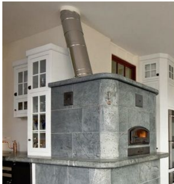
FIGURE 5.9. An example of a chimney offset from a heater to a desired location for travel through the rest of the house and through the roof. Heater by New England Hearth and Soapstone.
