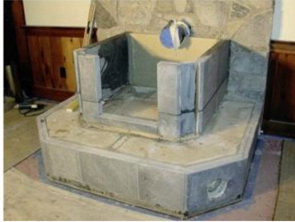
FIGURE 8.25. Following the rule that the container is built first, the next course of soapstone is erected. Note the continuing back wall of insulation board.
