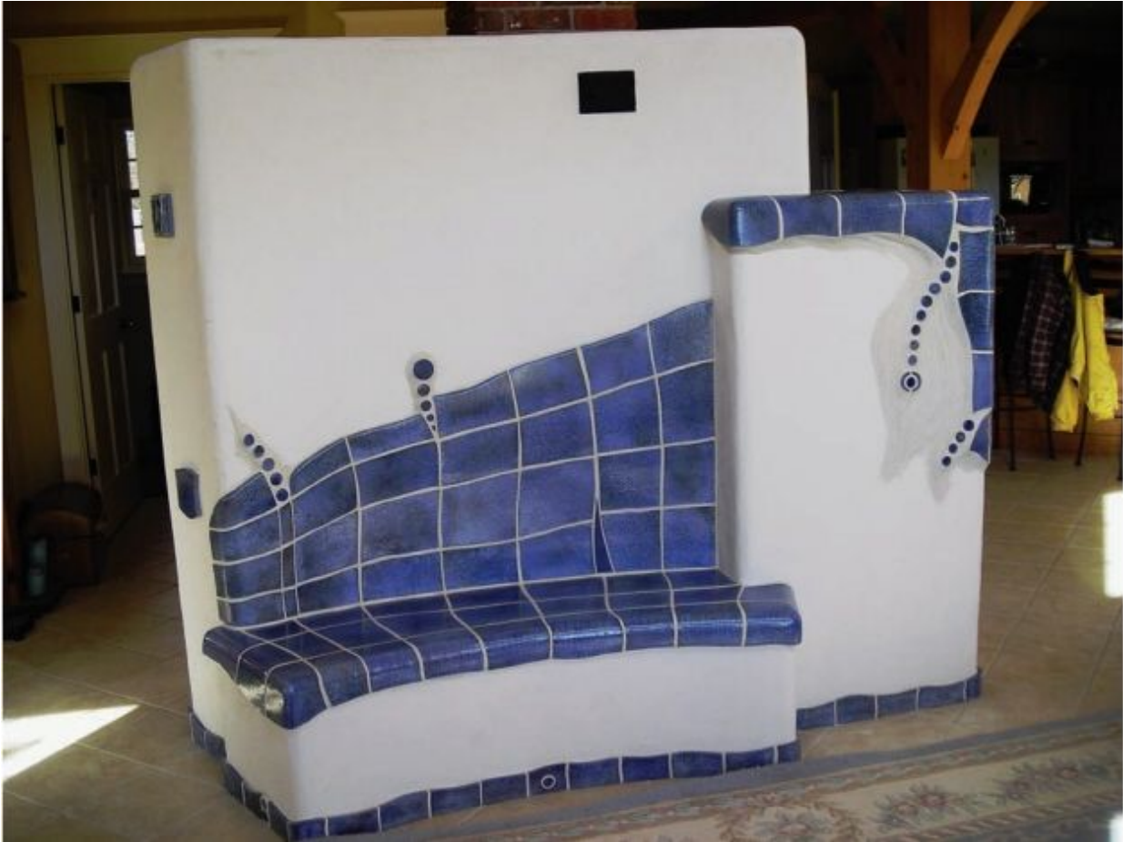
FIGURE 4.2. This heater was built using handmade tiles and stucco. Notice how the sitting area, which is heated, and the taller element have a gentle curve. Masonry heaters can have very organic shapes. Every surface visible here is a heating element. See the firebox side of this heater in figure 6.12. A kachelofen designed, built, and photographed by Ernst Kiesling, Canadian Kachelofen.
