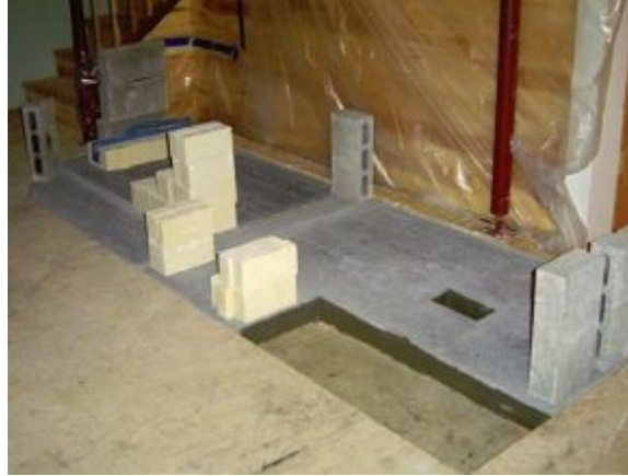
FIGURE 9.5. Foamglas, the charcoal-colored material, was laid on the foundation capping slab. Cement board was then bonded to the Foamglas. Photo by Julie Cline.
