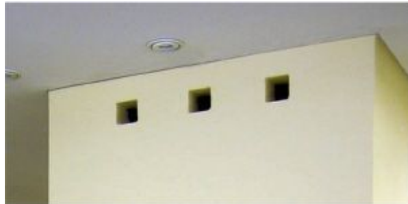
FIGURE 9.16. This heater is built tight to the ceiling. Square openings near the ceiling provide ventilation of the space. Without such provisions, heat accumulates around combustible framing members of the ceiling. Designed and built by Stovemaster; photo courtesy of Alex Chernov.
