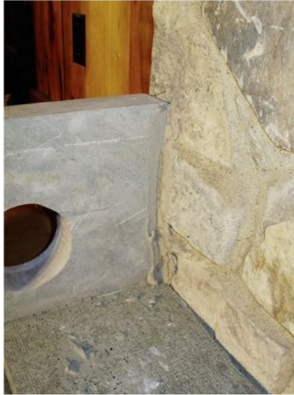
FIGURE 8.13. The first course of soapstone is custom-shaped to fit the existing stone wall. The stone wall is a veneer on a wood-framed wall and should be insulated from the inner life of the heater. Visible is the circular cleanout opening for access to the heated bench and the heater's first flue—a down flue from the firebox.
