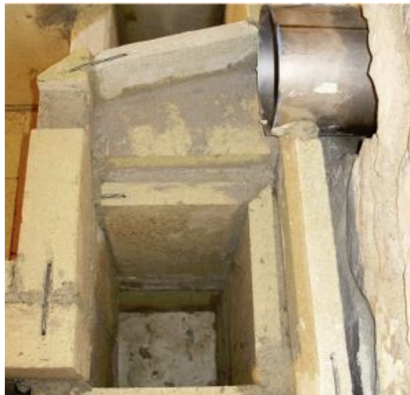
FIGURE 8.33. A view of the updraft vertical channel coming from the heated bench. Note the corners of the mitered refractory plates visible just under the opening of the steel flue. Again, mitered joints assure that the parts of the flue cannot fall inward during expansion and contraction. Pins or clips are unnecessary where such a mechanical preventive measure is taken.
