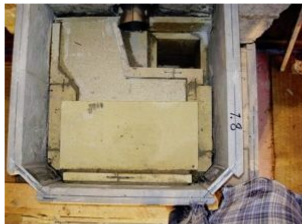
FIGURE 8.37. Thick 21.2-by-12-by-24-inch refractory slabs cover the insulation board and will create the surface on which the upper flues are built. These slabs do not rest on the insulation board, which is set dry (without mortar). The slabs span the insulation and rest on the other firebrick pieces pinned together on either side of the insulation board.
