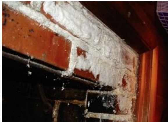
FIGURE 11.5. It may look like mold, but it's just a structure of minerals, called efflorescence, "growing" on the bricks as they dry. Photo courtesy of Charles Buell Inspections, Inc.
