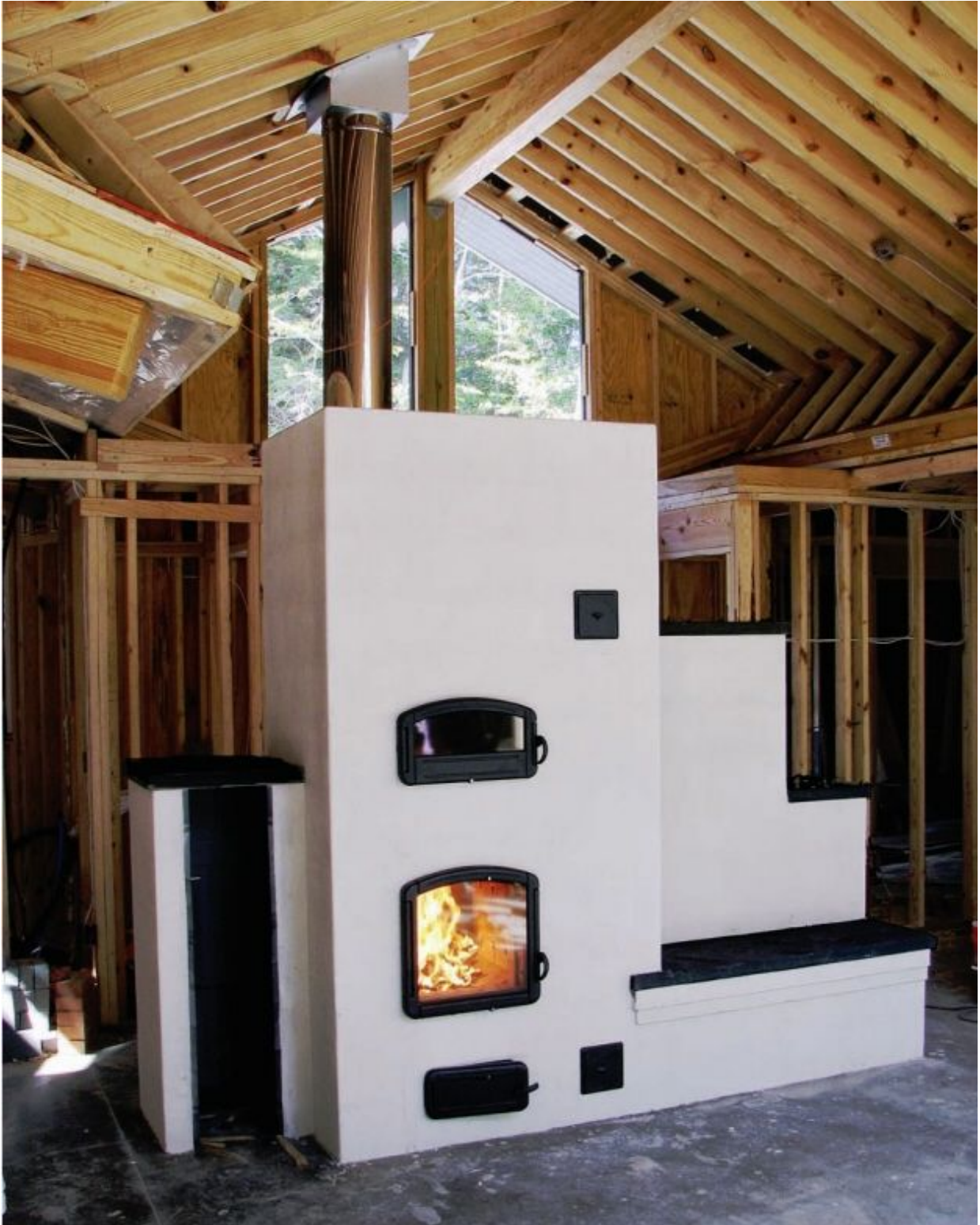
1. Plan for the chimney to be located within the heated confines of the home.
