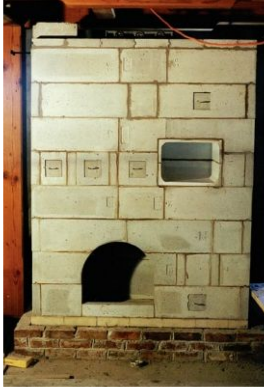
FIGURE 8.66. A completed Envirotech Radiant Fireplace core kit. The entire inner life is cast blocks of refractory concrete. Project by Masonry Heater Store; photo by Wendell Short.
