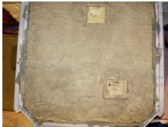
FIGURE 8.50. Once all the caps are installed, the entire “lid” is parged with clay mortar reinforced with fiberglass mesh. The mesh is again coated with clay to make a solid clay seal at the top of the masonry heater. The mesh is a reinforcement to add strength to the assembly. Two cleanout doors are set in place with clay mortar but left free of clay over their tops for future access.
