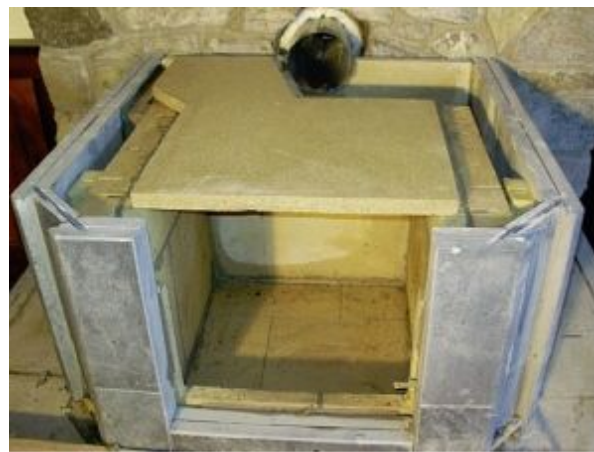
FIGURE 8.35. The firebox and first flue are covered with "hot face" Skamolox insulation. Insulating the ceiling of the firebox ensures that high combustion temperatures are maintained for maximum combustion efficiency and, therefore, clean emissions.
