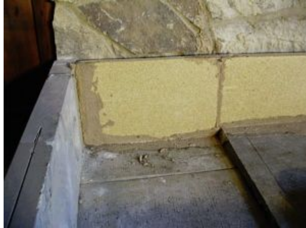
FIGURE 8.14. Skamolex insulation creates the back wall “veneer” of this heater, limiting heat transfer to the combustible wall behind the stone. The insulation board is set in clay mortar.
