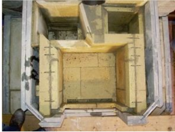
FIGURE 8.34. A full-plan view of the completed firebox, two rear vertical flues, the outburn, the gas slot, and flue exit. Note the 2-inch air space on either side of the firebox. This large space provides enough volume that a convective heat transfer will take place between the hot firebox walls and the soapstone veneer.
